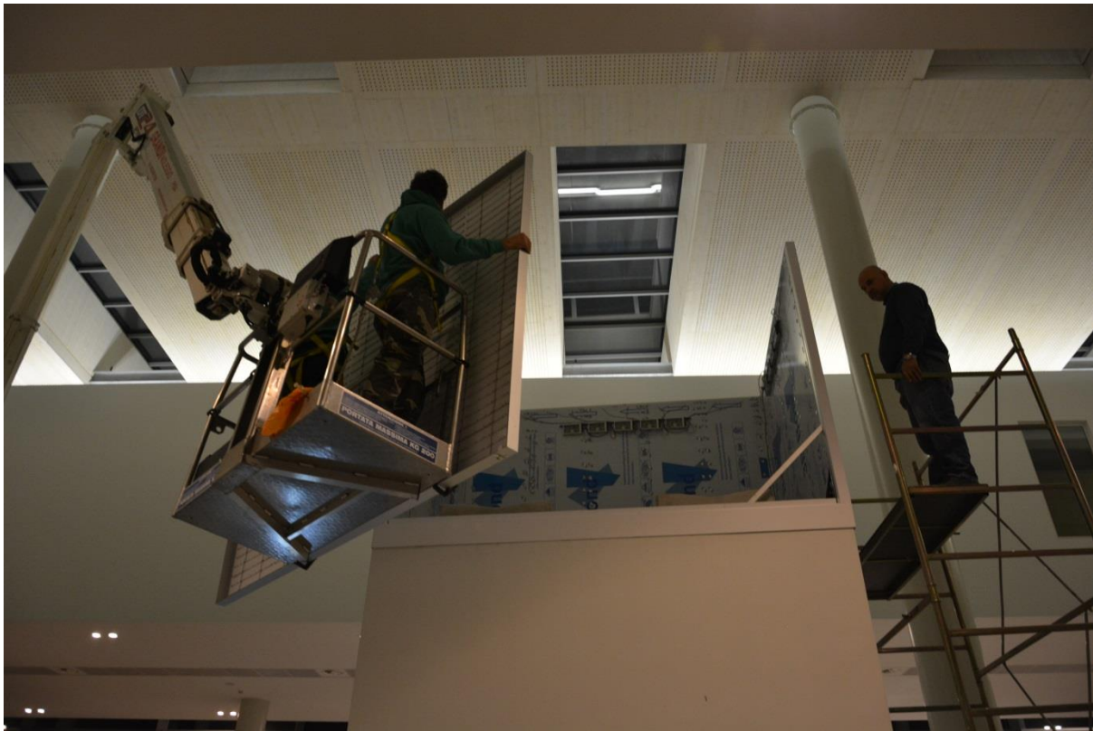
The advertising sign is going to be mounted above the tower lift.
